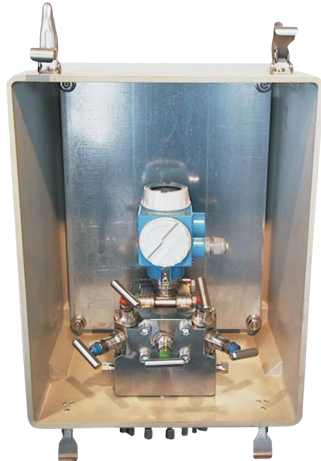
P5/ L style manifold in hard enclosure with transmitter mounted
